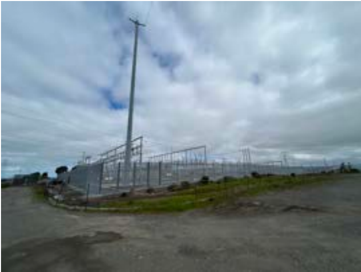
View C: PG&E Ravenswood Substation from Bay Trail facing north.
